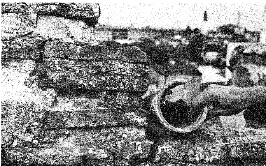
Fig. 6. Example of a true Ottoman dome built of brick and equipped with rows of pots to absorb reverberation. Dikkancik Cami 1550/51, Skopje, Jugoslav Macedonia..
